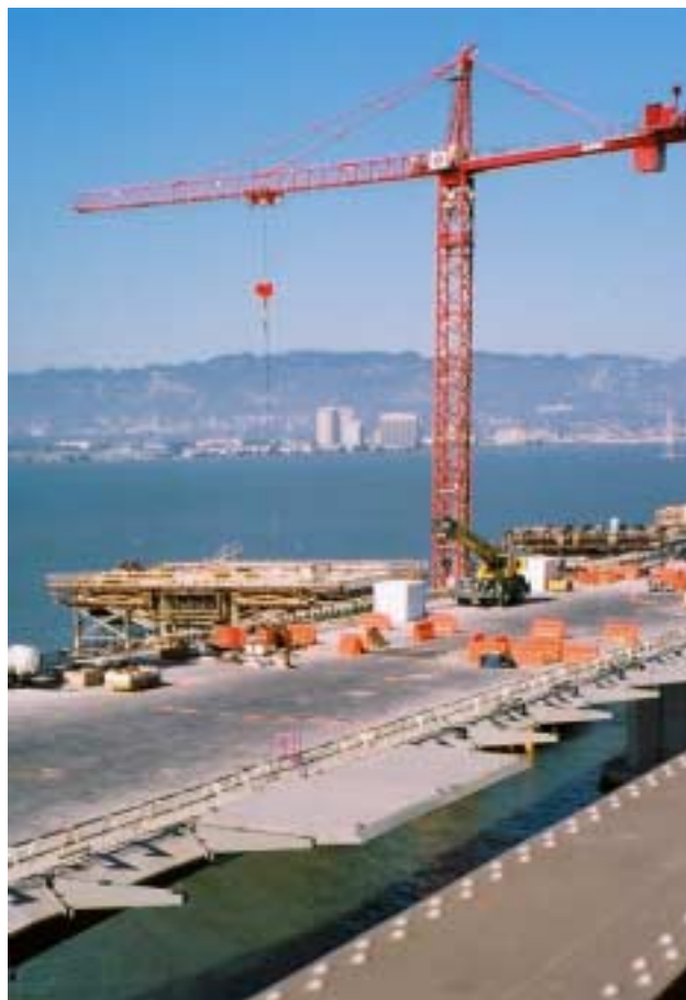
View of new East Span under construction. The first decks of the Alex Zuckerman East Span Bikepath are attached to the support beams.
