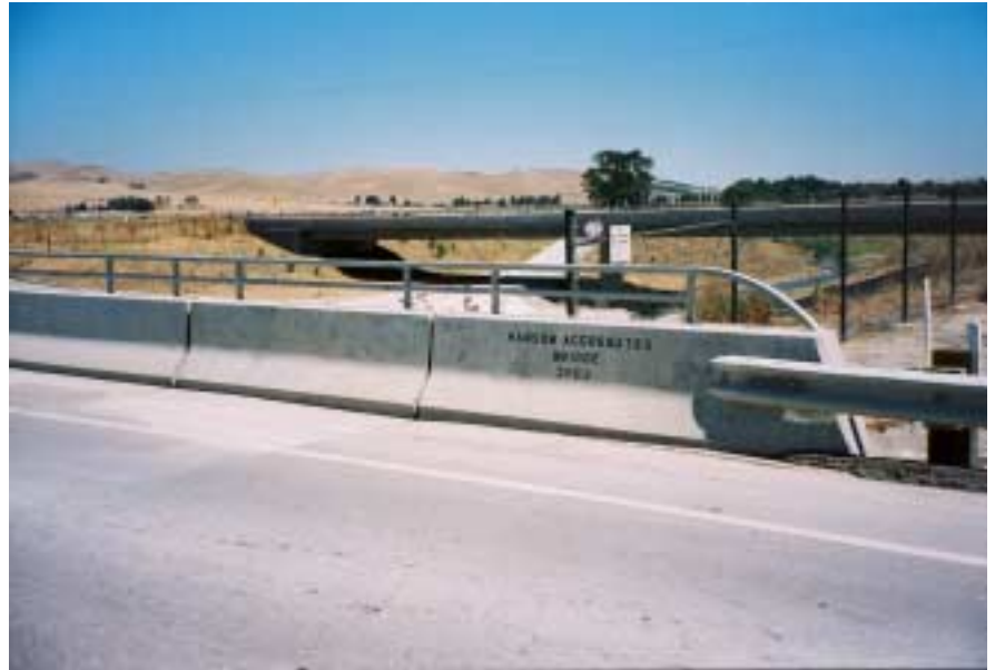
Unused bridge to the abandoned Hanson quarry site could become the junction for two trails connecting Pleasanton with Livermore.
